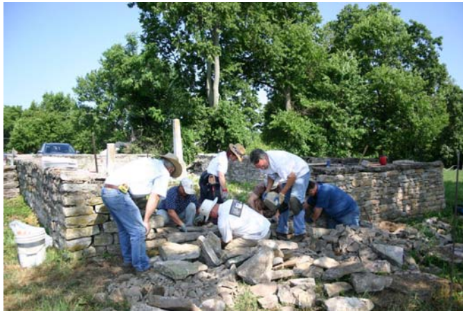
Master Craftsman David Kenley led a group of volunteers who helped restore this cemetery fence at Great Crossing Baptist Church in Scott County.
